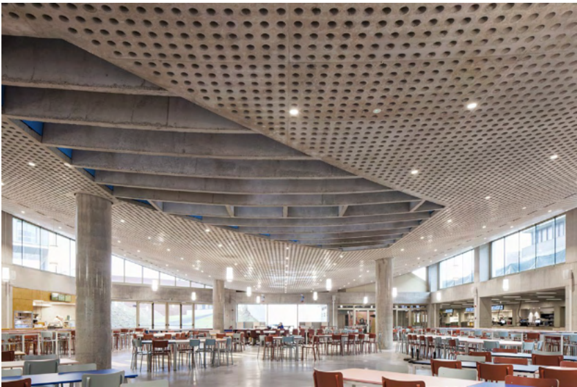
The perforated concrete ceiling in the Alma of Gasthuisberg (Leuven, Belgium). Photo by Johnny Umans.
