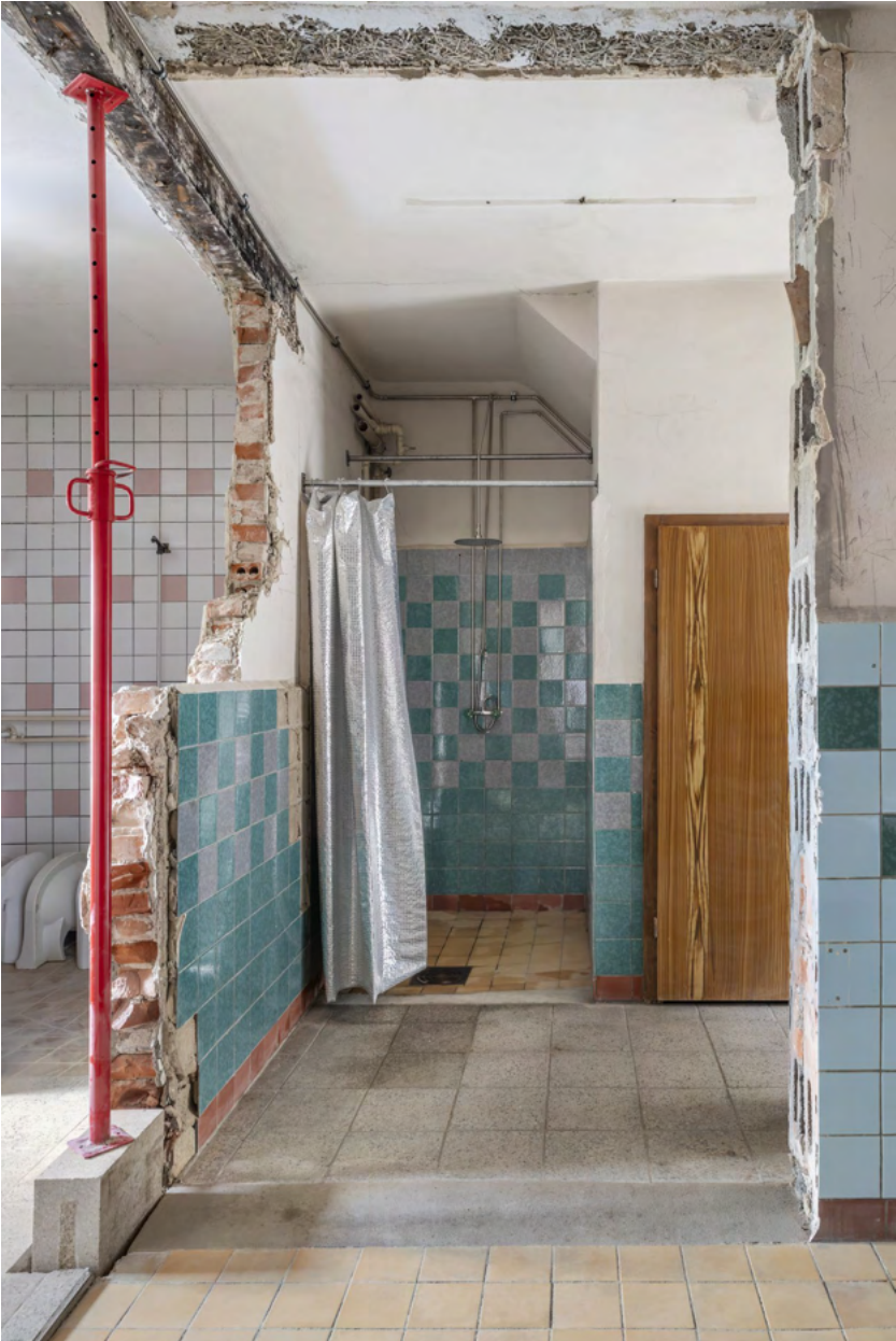
fig. 1 11th of July 2025 - End of the design and construction phase in the summer semester 2025, showing the intermediate state of the bathroom with a functioning shower and a barrier-free toilet. ©Hannes Heitmüller
