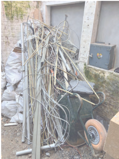
19.03.2026—JDB (image credit: Bratco BV) Collected cables and conduits for possible later reuse are stored in the courtyard.
