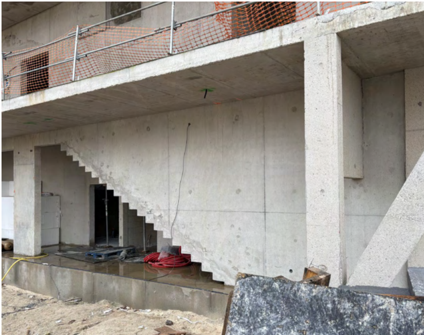
Construction site halted at the structural shell stage, March 2026. Photography: Florian Buquet.
