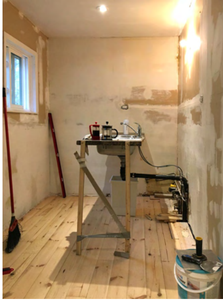
Image 8: Kitchen, for about three weeks, in our continual, lived-in construction site. Kids said, about the kitchen, “it was fine”.
