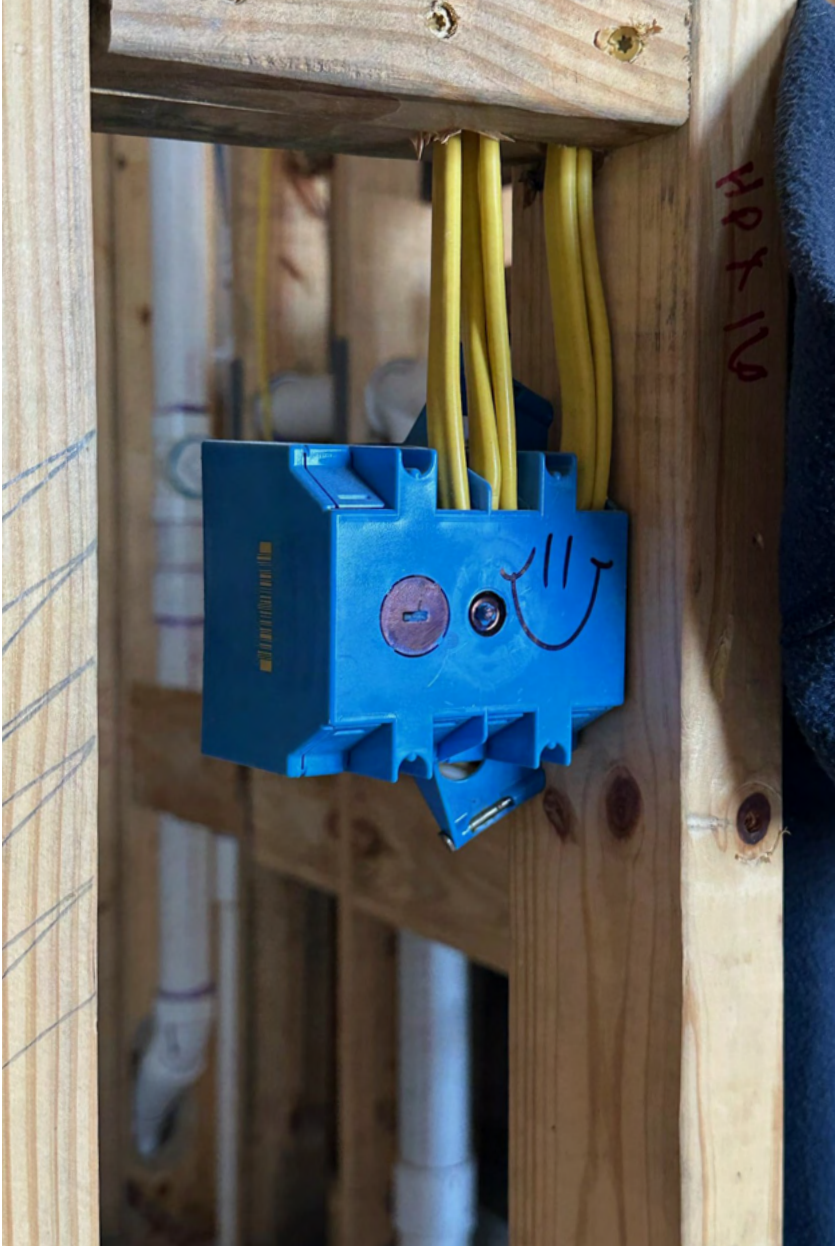
Fig. 4 A smiley face drawn on a blue electrical junction box connected to yellow cables, mounted on wooden stud
