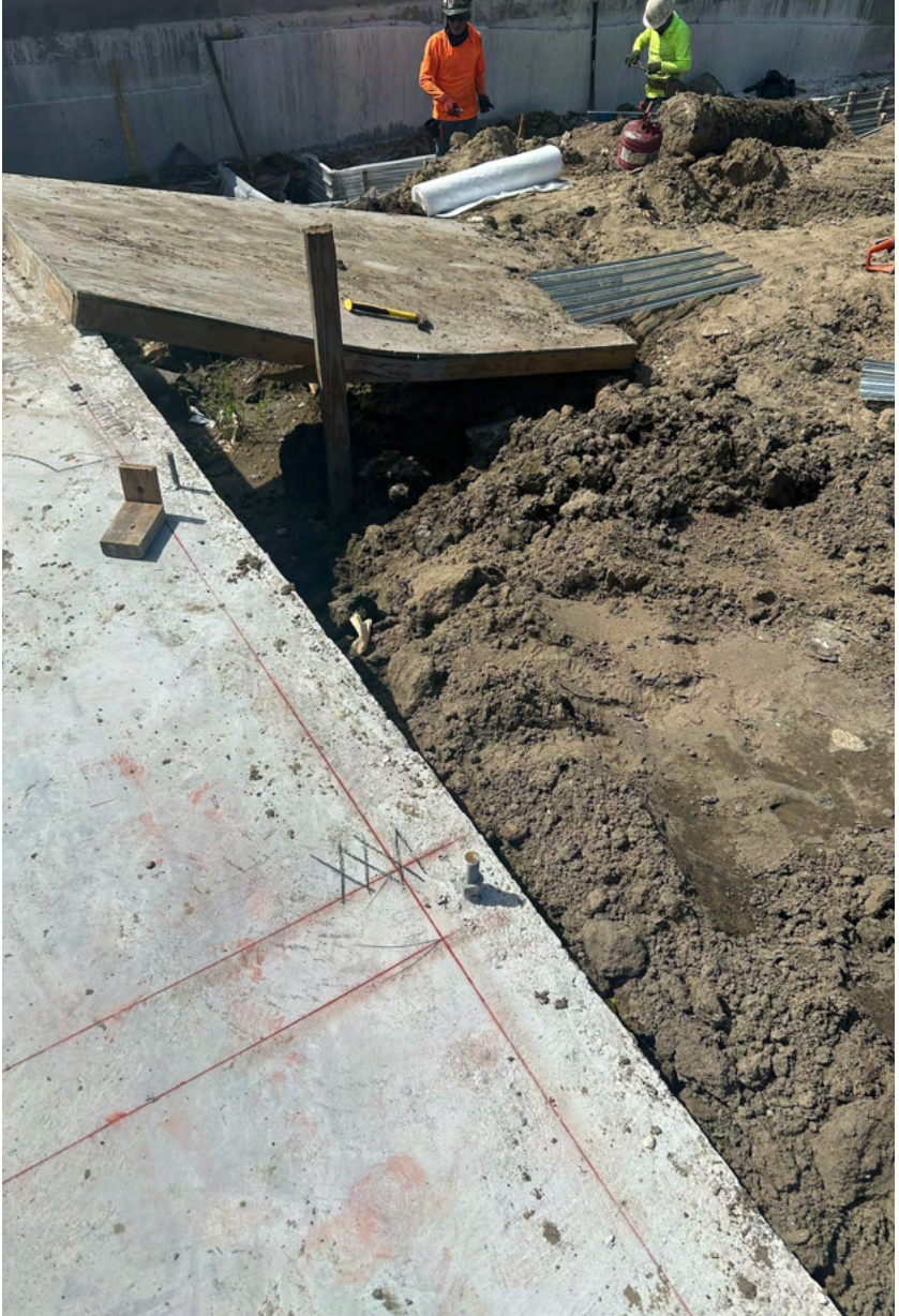
Fig.8 1 to 1 scale framing layout on concrete slab. "X" indicates stud framing while red chalk indicates the width of the wall.
