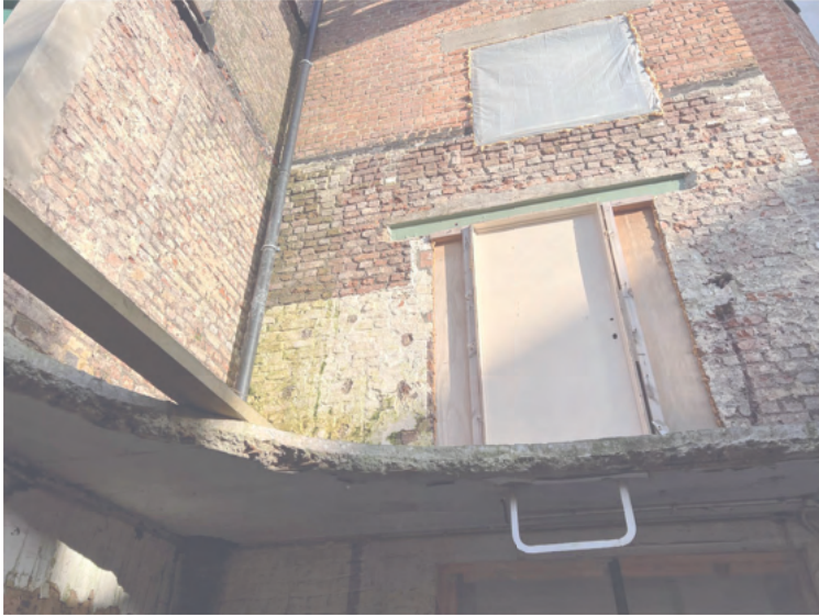
05.03.2026—JDB (image credit: Bratco BV) A new slab opening in the courtyard.
