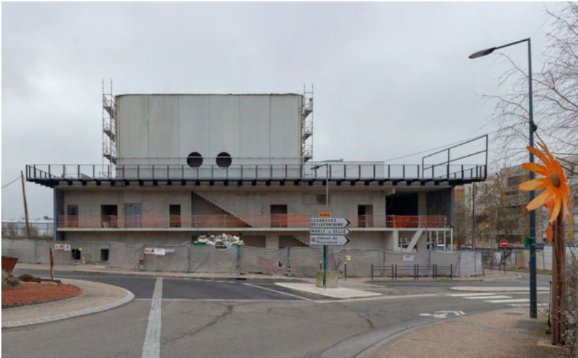
Construction site halted at the structural shell stage, March 2026. Photography: Florian Buquet.
