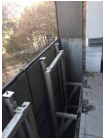
280 Smit Street (Top to Bottom) 2015, Intact Window 2016, Window Removed
